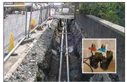
Heating main used in community heating systems
