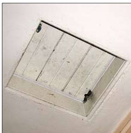
Loft access cover with draughtproof and lock
